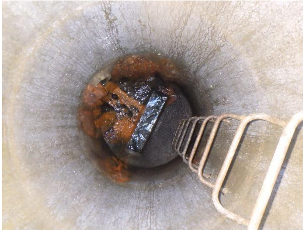
Infiltrations – Site Chavany
